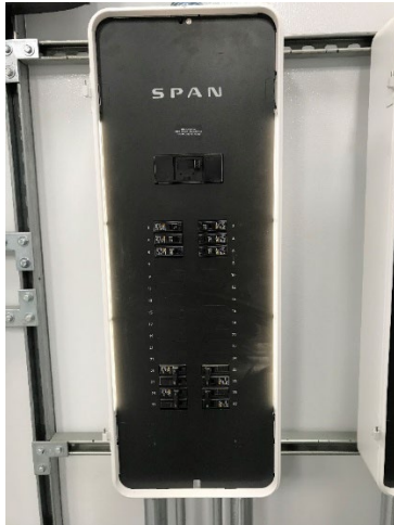
SPAN Panel Unit Under Test
