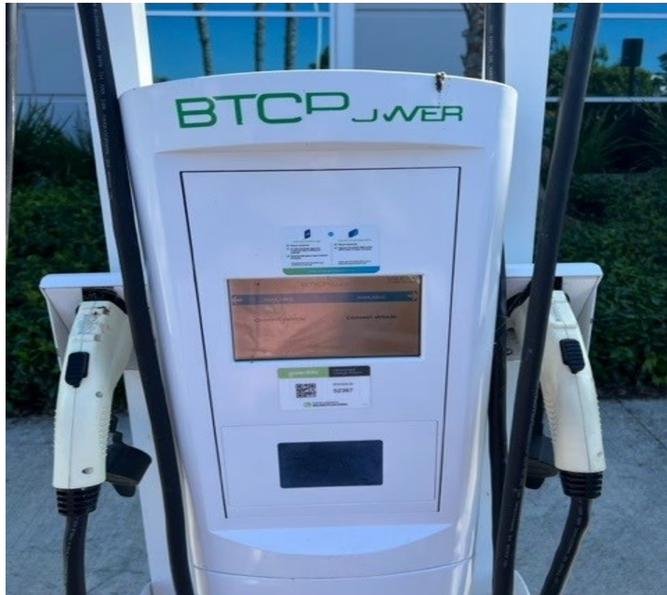
FIGURE 4. BALFOUR EV CHARGER WITH GREENLOTS NETWORK
