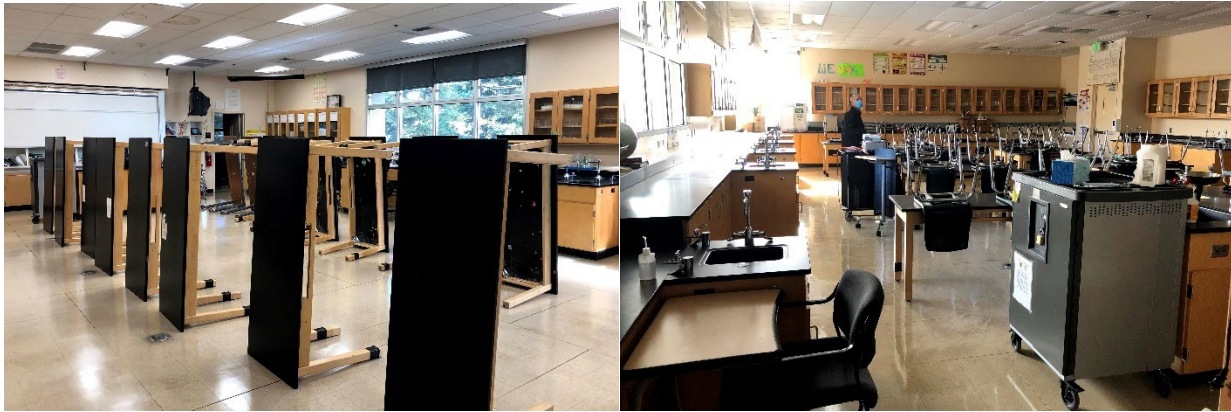
FIGURE 6. CLASSROOM SERVED BY BASELINE RTU (LEFT) AND CLASSROOM SERVED BY PACKAGED HEAT PUMP WITH IDEC (RIGHT)
