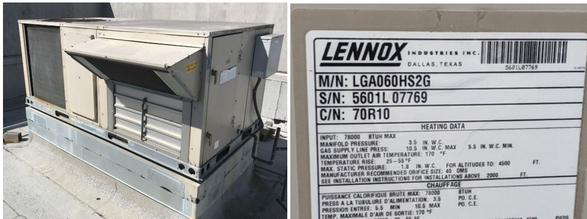
FIGURE 4. BASELINE LENNOX 5-TON RTU
