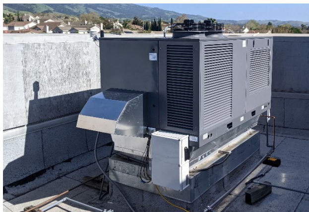
FIGURE 5. PACKAGED HEAT PUMP WITH IDEC RTU
