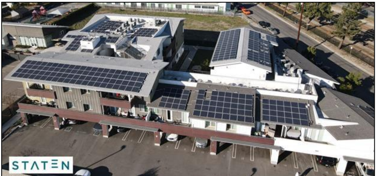
Aerial View of the Willowbrook PV Installation
