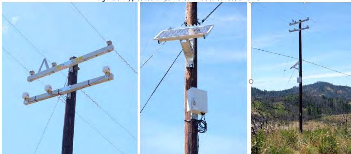
Figure 9. Typical solar-powered RF data collection unit
