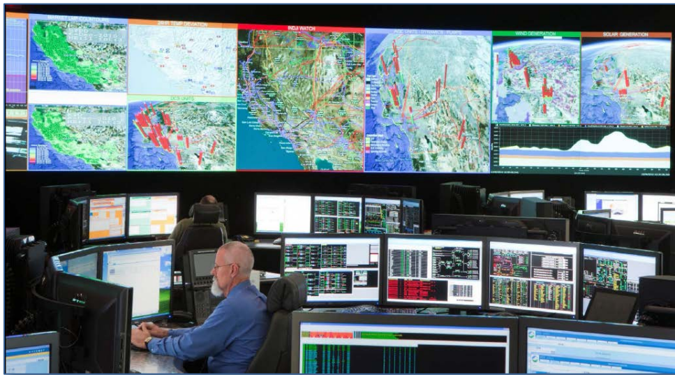
Figure 8: CAISO Control Room Tracking Renewable Profiles
