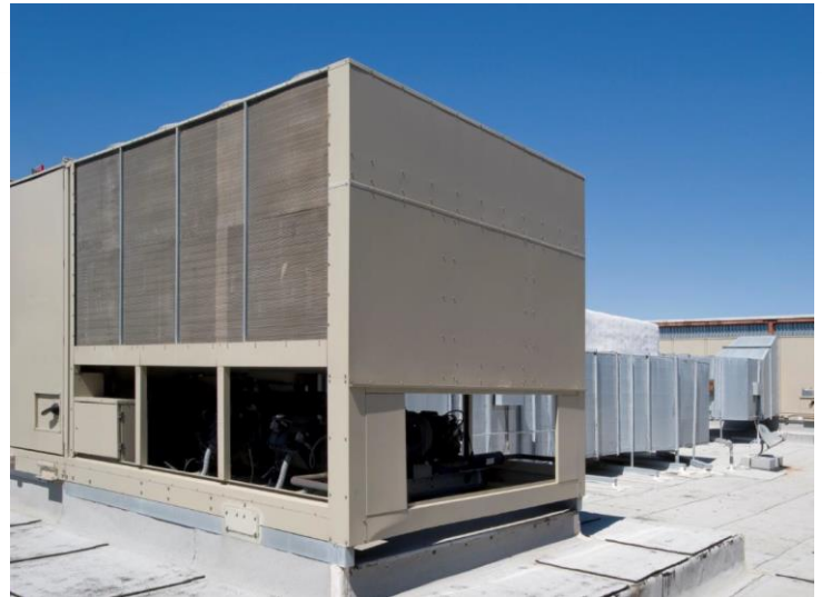
Image 1: HVAC Unit on Commercial Building
