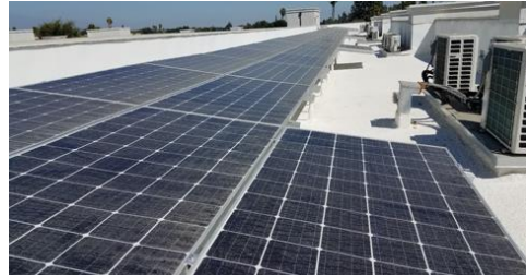
Figure 11: Solar PV Array
