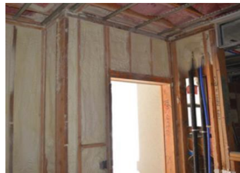
Figure 9: CCSF Foam Insulation
