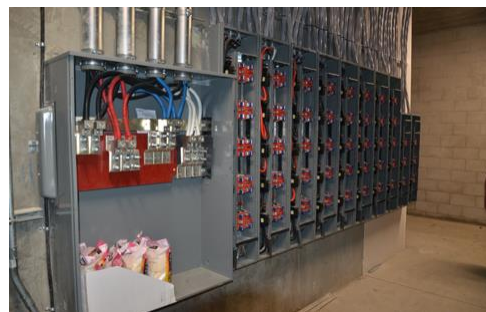
Figure 12: Meter Base for the 46 Apartments
