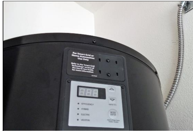
Figure 4-8 Communications port provided by water heater
