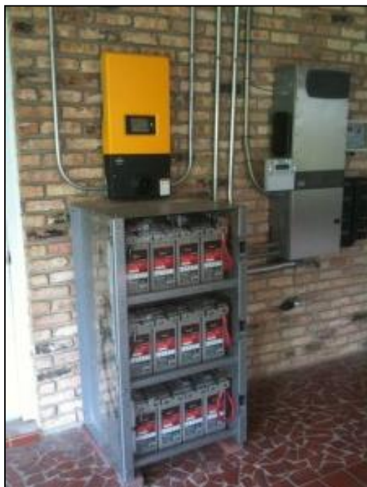
Figure C-12 An Outback Power installation with lead-acid batteries.
