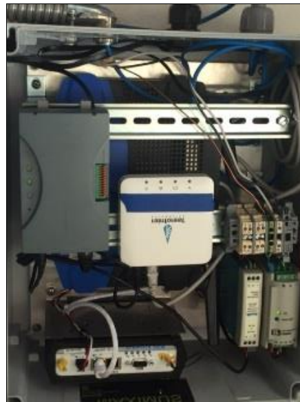
Figure 4-11 Data box installed in each of the 20 sites
