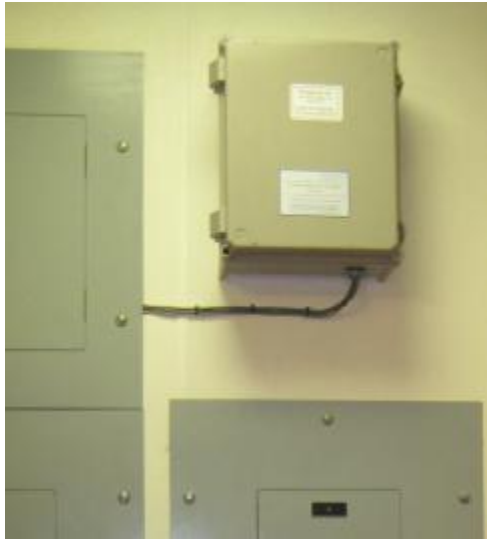
FIGURE 2. K20 POWER LOGGER MOUNTED NEXT TO ELECTRIC PANELS
