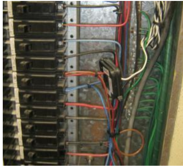
FIGURE 3. CURRENT TRANSDUCER MOUNTED INSIDE ELECTRIC PANEL
