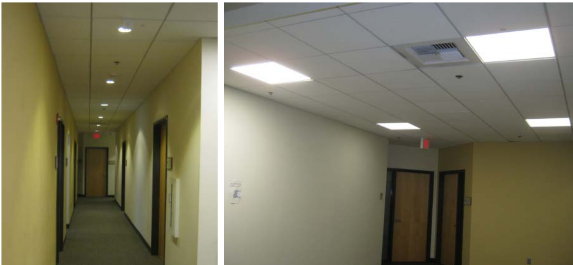
FIGURE 3. STRAIGHT CORRIDOR LED CAN LIGHTS (LEFT) AND 2X2 LED LOBBY LIGHTS (RIGHT)
