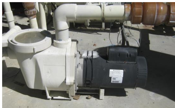
FIGURE 9. MOTOR ON/OFF LOGGER STRAPPED TO TOP OF MOTOR
