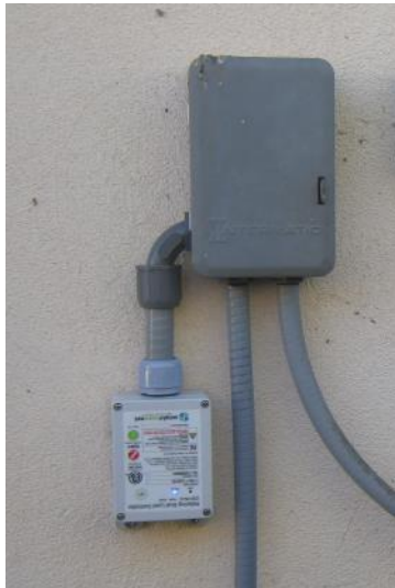
FIGURE 2. SYSTEM 1 LOAD CONTROLLER
