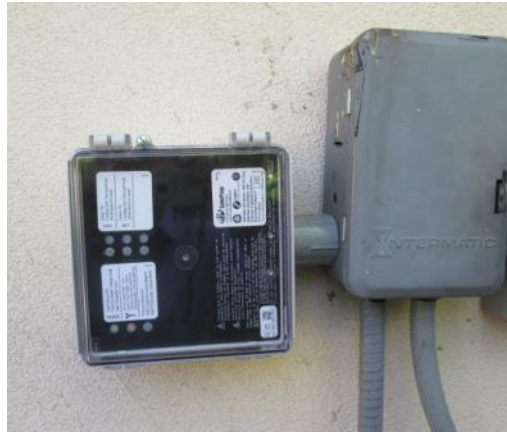
FIGURE 4. SYSTEM 2 LOAD CONTROLLER
